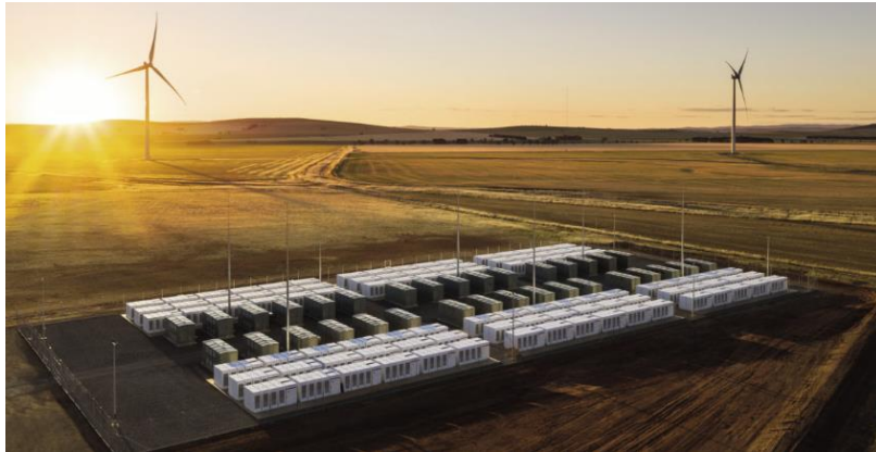
Figure 9. The world's largest 100 MW/129 MWh lithium-ion battery in Hornsdale, South Australia. [35](Source: Tesla)
